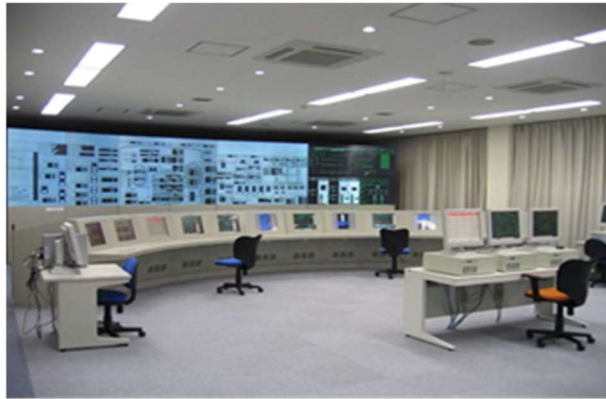
Figure 2. Digital Control Room
