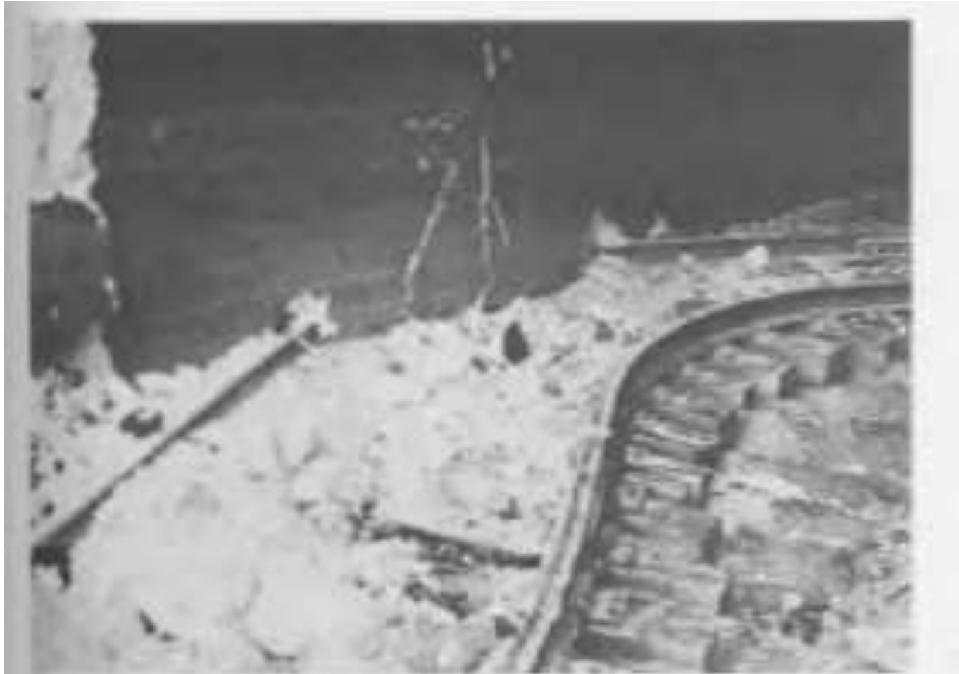
FIGURE 5. Damage near the east portal of tunnel 3. Apparently the wall was raised just as the truck bent, and the wall then came down on top of the rail. View northwest.
