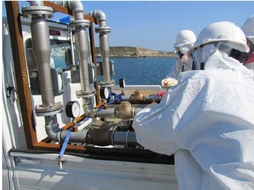
Injecting water to temporary headers, designed to practice connection to feed water pipes
