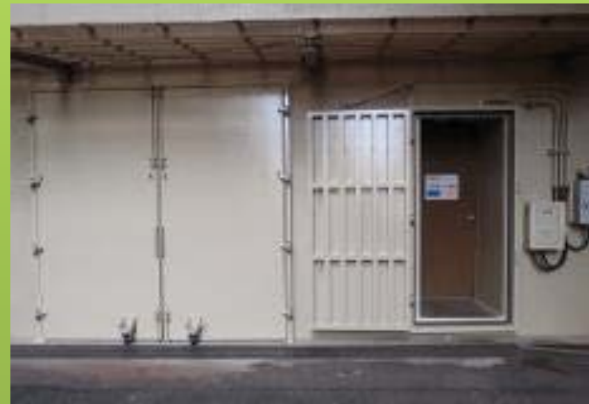
Watertight door that prevents water intrusion into safety significant buildings
