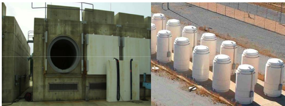
Figure 1: Horizontal Dry Storage (left) and Vertical Dry Storage (right)
